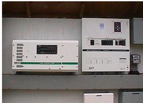
An inverter (left) and charge controller (right) are the power conditioning components of a PV system.
